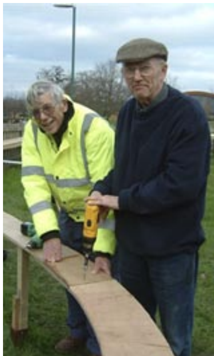
Gordon Miles and Dave White screw the final piece of plywood in place. Now they have to cover it all with roofing felt.
